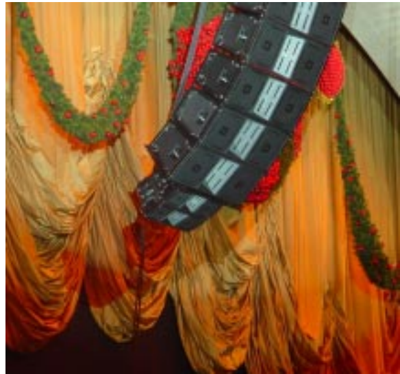
Two compact VT4887 speakers for front fill are hung under the main array of fifteen VT4889 speakers.
