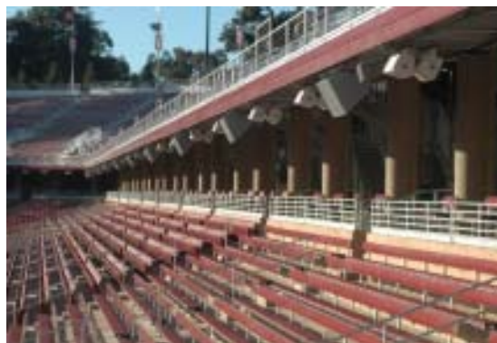
Pro Media/Ultrasound installed an audio system comprised of JBL PD Series, AM Series and Control Contractor Series loudspeakers at the new Stanford Stadium.
