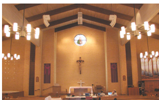
Electro Acoustics designed and installed a JBL VRX line array system for St. Paul the Apostle Church in Richardson, Texas.
