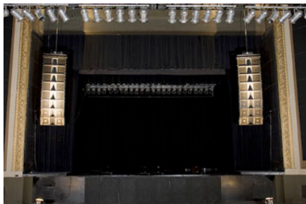
The renovated Rialto Theatre in Tucson, Arizona features a new JBL VERTEC® line array system.
