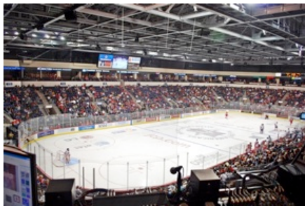
Daktronics installed a JBL AE Series loudspeaker system at the Allen Event Center in Texas.
