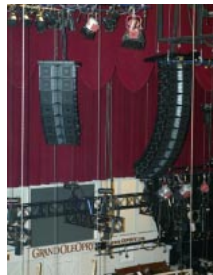
The 4,400 seat Grand Ole Opry House's new JBL sound system includes VERTEC line arrays, driven by Crown MacroTech power amplifiers.
