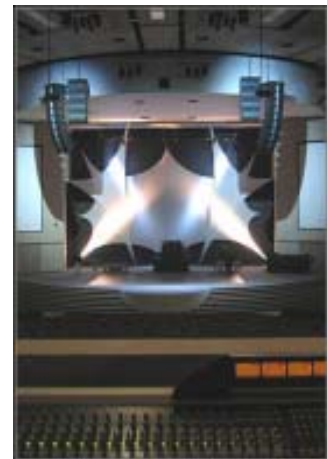
A VERTEC DP Series line array system was recently installed at the Moreleta Park Dutch Reformed Church in Pretoria, South Africa.
