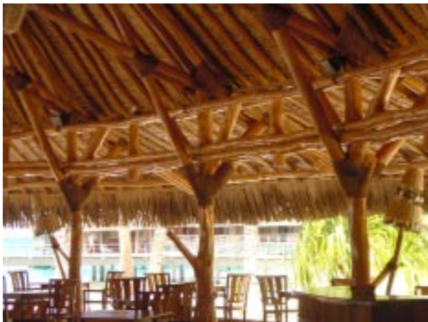
Control Contractor speakers installed in the outdoor grill
